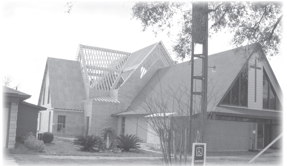
St. Joseph Church in Inez doubles its capacity to seat 400 people. The completion is expected around late summer.
