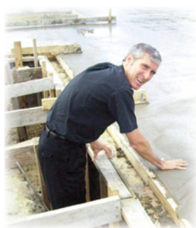
Father Gary, pastor of St. Philip Church, makes a handprint in the cement foundation of the school's new gym.
