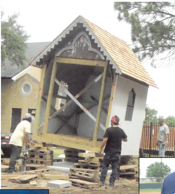
The future Marti Love Chapel is lowered to the ground at its new location, which very well may be its original location. It was returned from the former Stanzel home to St. Rose of Lima Church to be renovated. The blessing of the chapel will be held Sept. 30.
