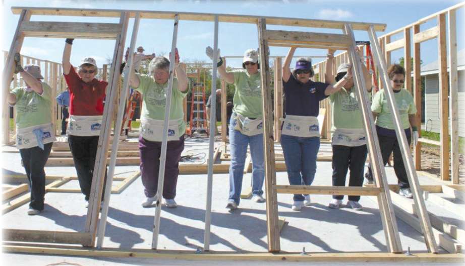
(below) CDA chairmen and deputies raise a wall on the 5th Habitat State Build home.
